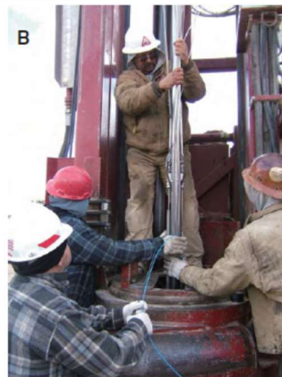
Figure 4. [A] Borehole NC-EWDP-24PB completion schematic showing permanently installed U-tube samplers using alternating levels of sand and ben/sand backfill. [B] Running-in-hole with U-tubes and DTPS sensor being strapped onto a central 2" stainless steel piezometer.
